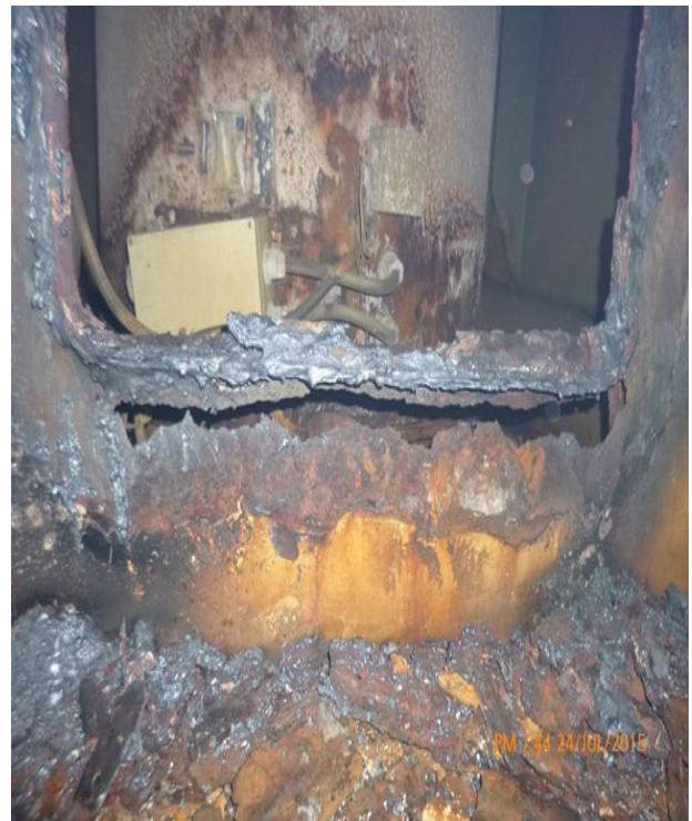
Condition of bottom part which required replacement
