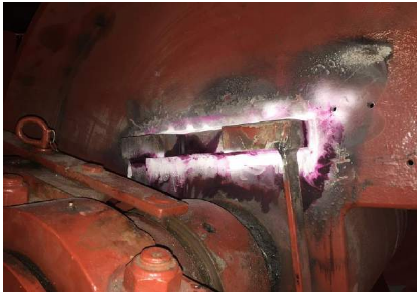
↖ ↗ Upon completion, ship crew carried out one coat of primer on new refit support section.
