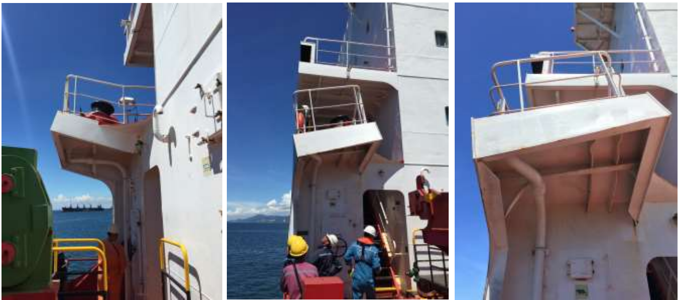
Inspected damaged location with Surveyor & discussed through repair procedure
