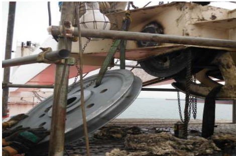
lifted new spare sheaves in position for alignment. Pin were kept 4 hours in ship's freezer and transfer to the crane jib by ice box.
