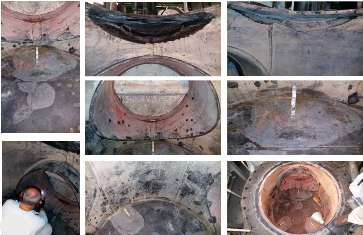
After cropped off the damages Chief Engineer were witnessed the progress and found Satisfactory.
