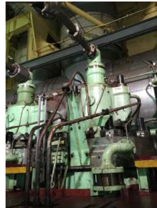
All connections are back in Place in good order
